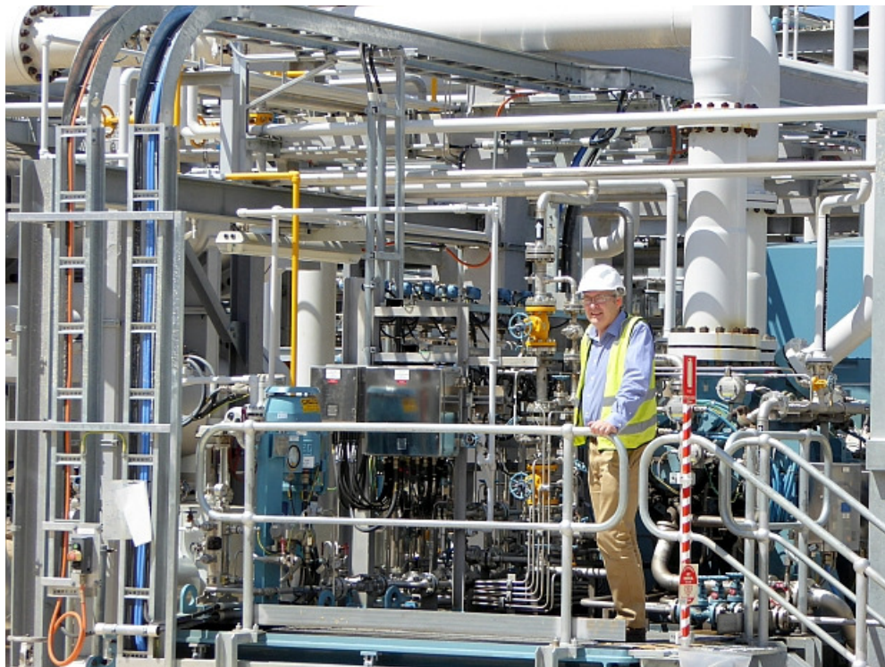
Richard Wawrzon at the base of a refrigeration circuit.
